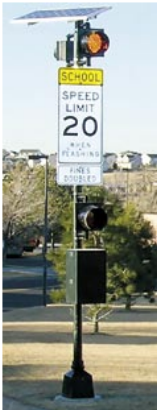
Painted Cabinet & Pole with Tattletale Light
