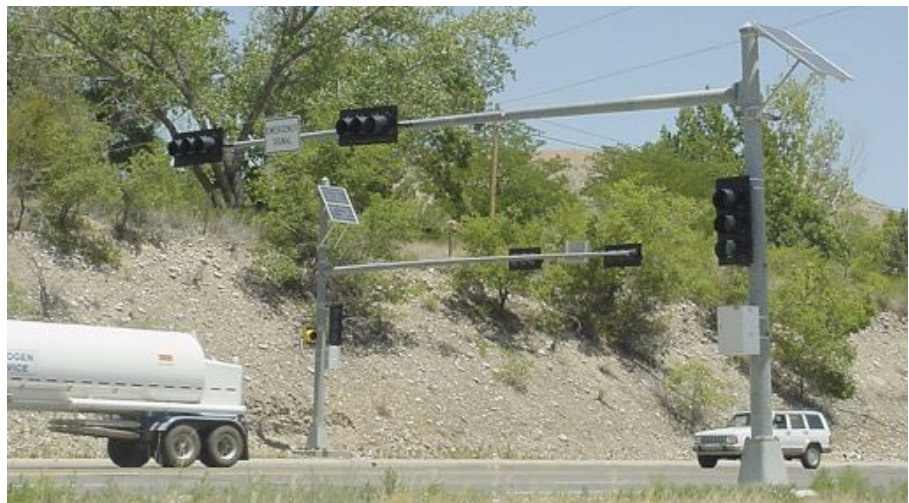
Three 3-section signal heads (solar powered). Lights are green until fire station activates.
